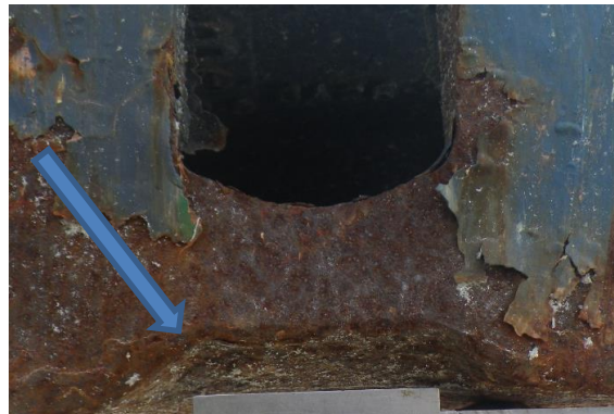
Action – Replace corner fitting – aperture shape and size altered
