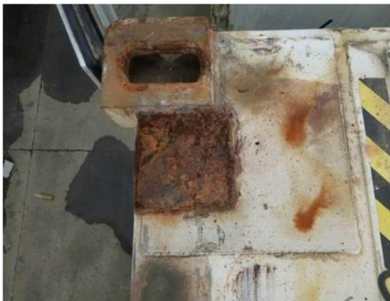
Non-conforming repair on Corner Protection Plate. Patch exceeds original size of Corner Protection Plate. Excessive corrosion likely due to poor coating applied.
