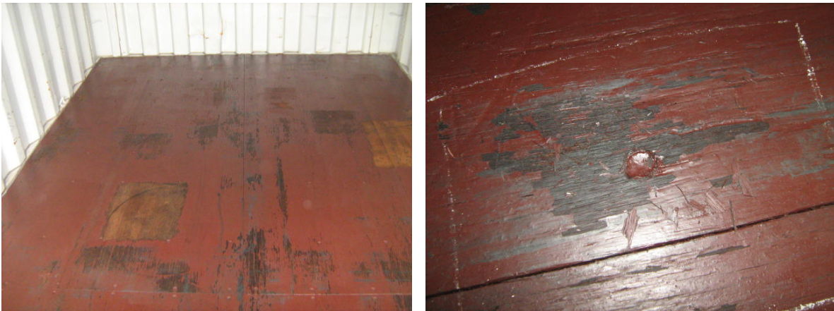
Examples of floor coating failure creating potentially unsafe conditions
