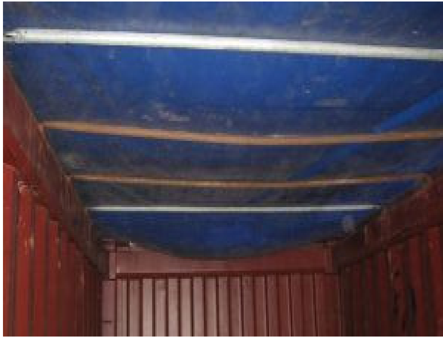
Improper bows Wrong material (not galvanized) No cammber
