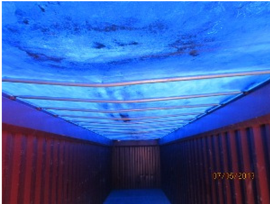
Roof bows to thin No camber
