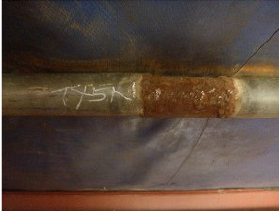
Improper Section Will cause tarp damage
