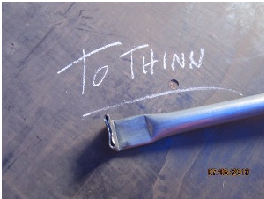
Improperly fitted roof bo end
